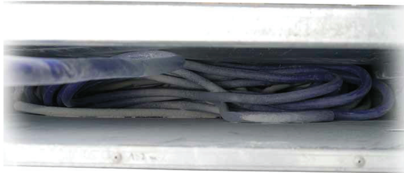
Fig. 7: Trailing cable in the cable bin
